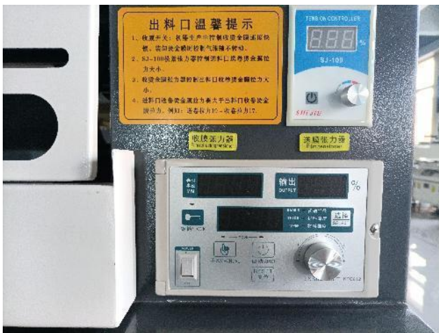
Discharge port control panel
